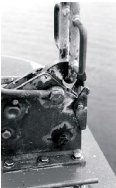
Photo 9. View of hook, suspension ring, and retaining latch
