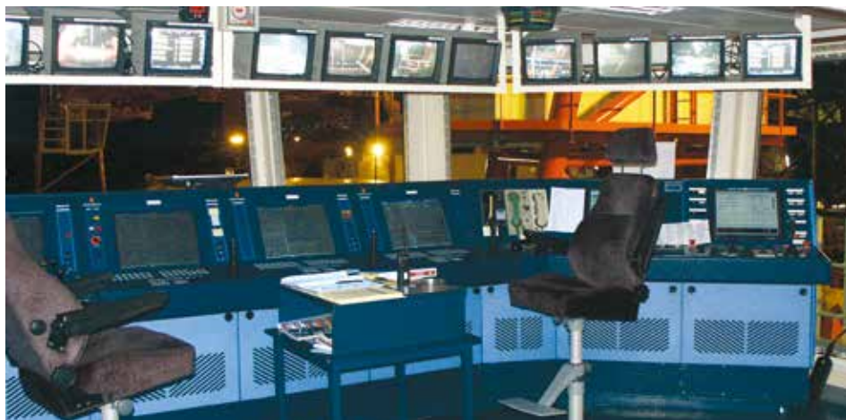
DP control station in offshore construction barge Balder
