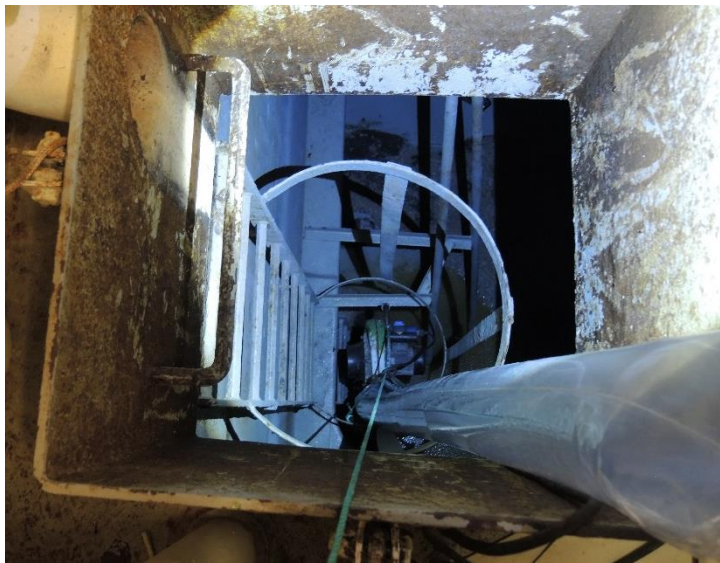
Figure 6: The ladder cage on the ladder in the silage tank obstructed the hoisting operation. Photo: AIBN
