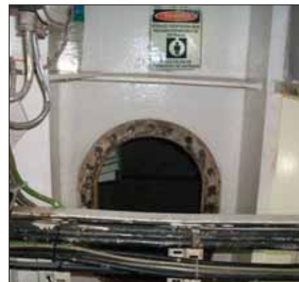
▲ This access is adequate but regrettably, the builders have put a cable run across the access
